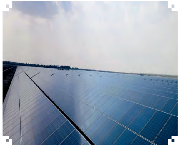
300 MW Solar power project set-up by Adani Solar Energy RJ One Pvt Ltd in Jaisalmer, Rajasthan
