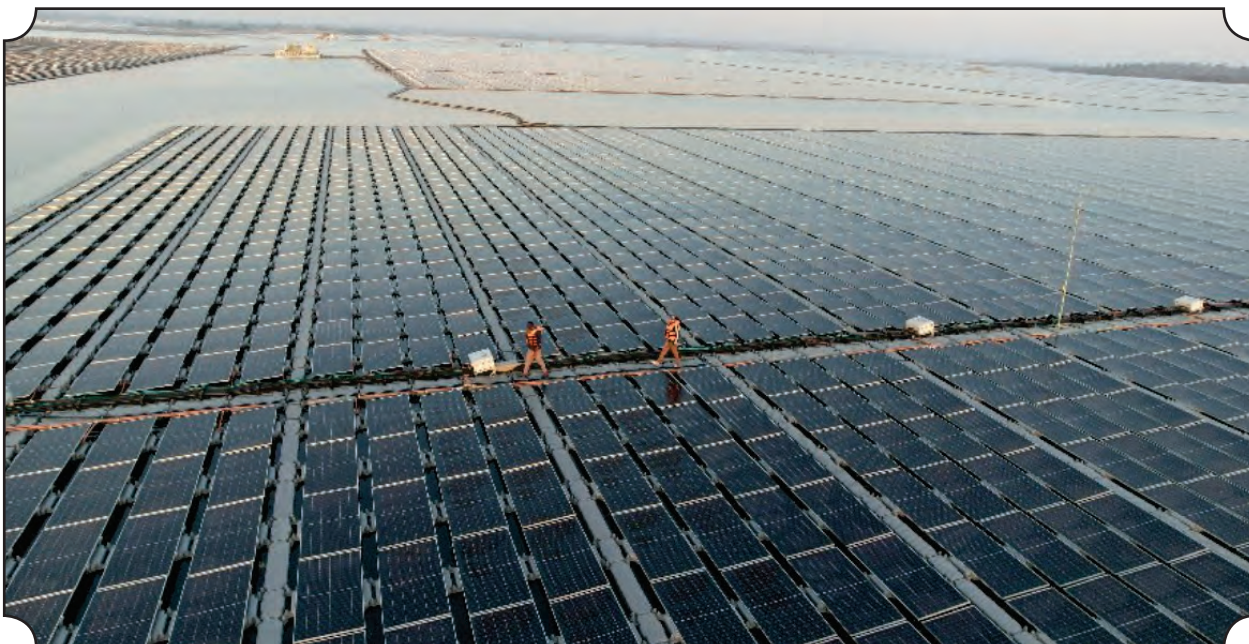
IREDA funded 100 MW Floating Solar power project set-up by AMP Energy Green Seven Pvt. Ltd. in Madhya Pradesh
