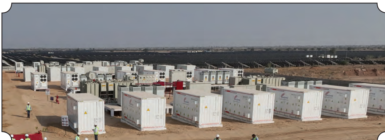
IREDA funded 300 MW / 601.9 MWh Battery Energy Storage System (BESS) at Pokhran, Jaisalmer, Rajasthan- IREDA's first merchant-based BESS project
