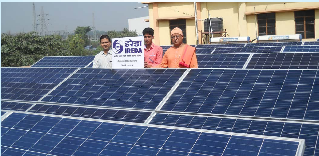
IREDA installed 75 kWp Solar PV System at R. K. Mission Ashram, Asansol under CSR Initiative
